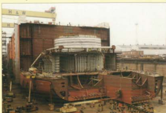
Construction of the Schiehallion FPSO in the Building Dock, clearly showing the lower section of the 14m moonpool. (January 1997)
